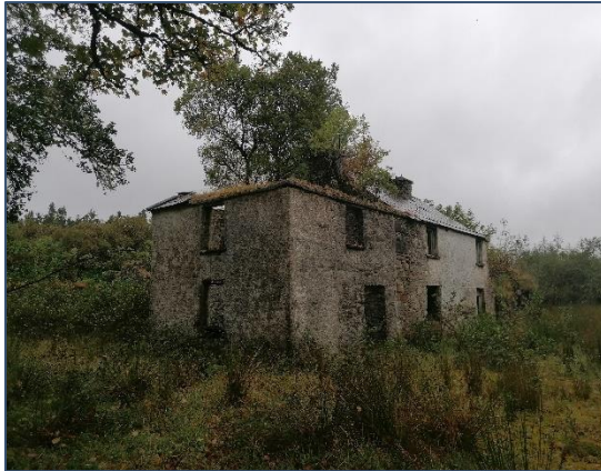
Plate 4-11 Derelict farmhouse with partial roof collapse
